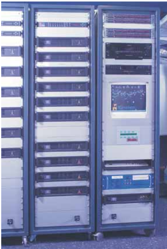
Racks with Amplifiers, DIPIT
